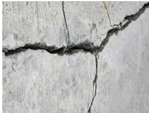
© stone crack, Fotolia #36569926
